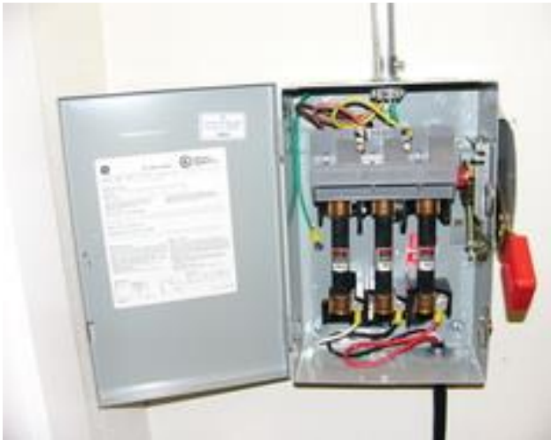
Ground wire should be connected to the cord
