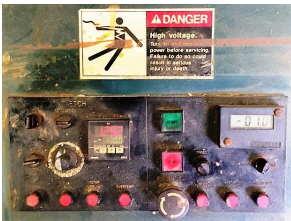
Splattered chemical on a control panel
