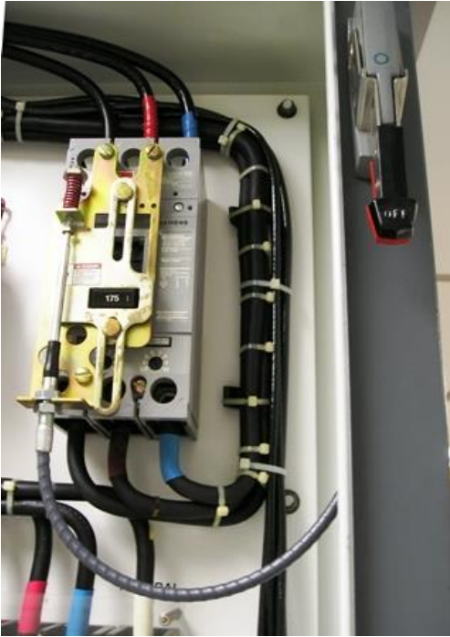
Disconnect can be a circuit breaker handle
