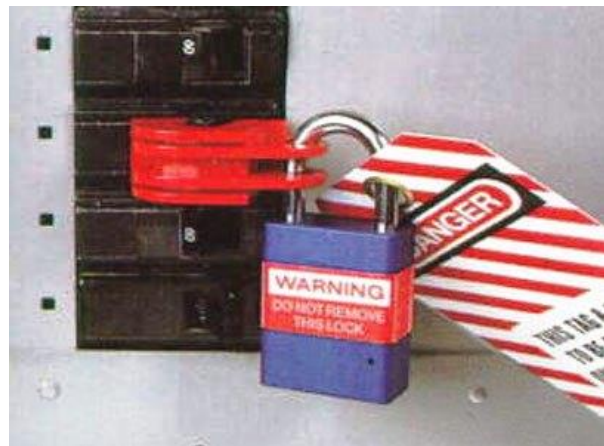
Cal-OSHA permits temporary clips for LOTO. NEC 110.25 states that portable locking mechanisms intended for temporary application are not acceptable for LOTO.
