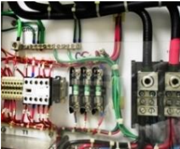
Neat and safe wiring with touchproof guard
