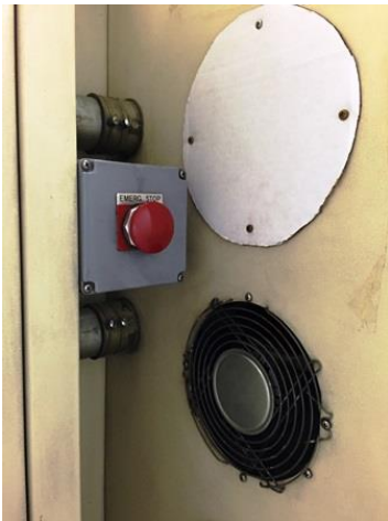
Check for dead and missing fans
