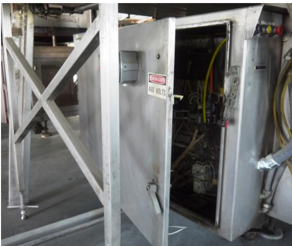
Inadequate clearance - door must swing 90°
