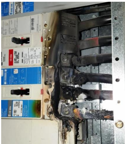
Loose terminals, then oxidation, then burn-out
