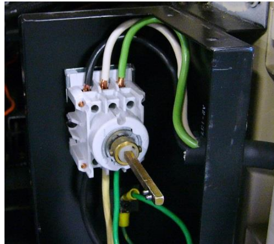
Ground wire should be permanent not switched
