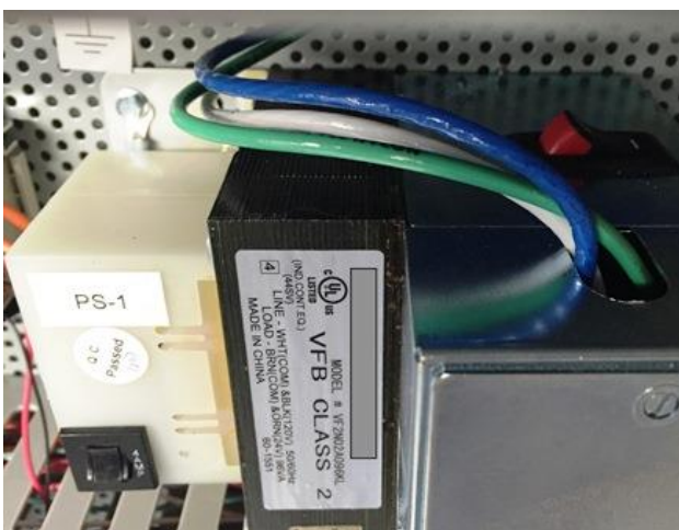
Hook-up across a sharp edge needs a grommet
