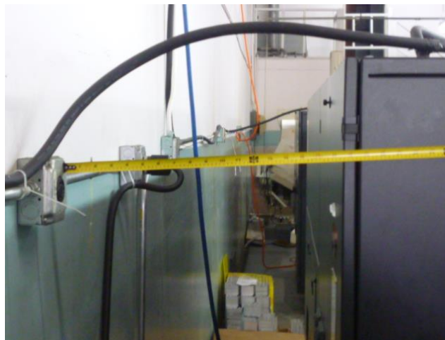
Inadequate clearance - must be 36 inches
