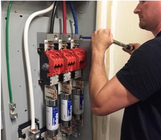
Good: wiring terminals torqued to spec
