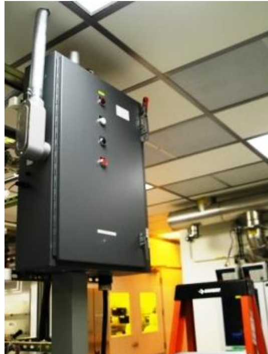
This disconnect switch is too high. It should be "readily accessible" and not require a ladder.
