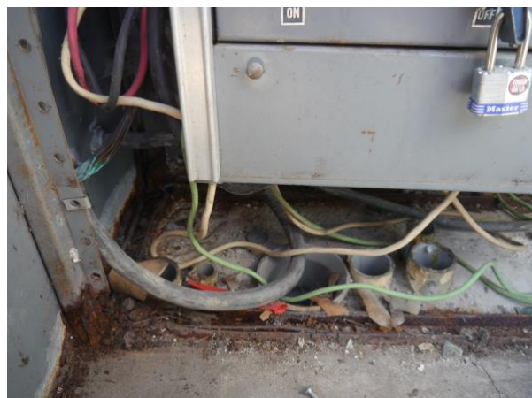
Corrosion on the floor of an outdoor panel
