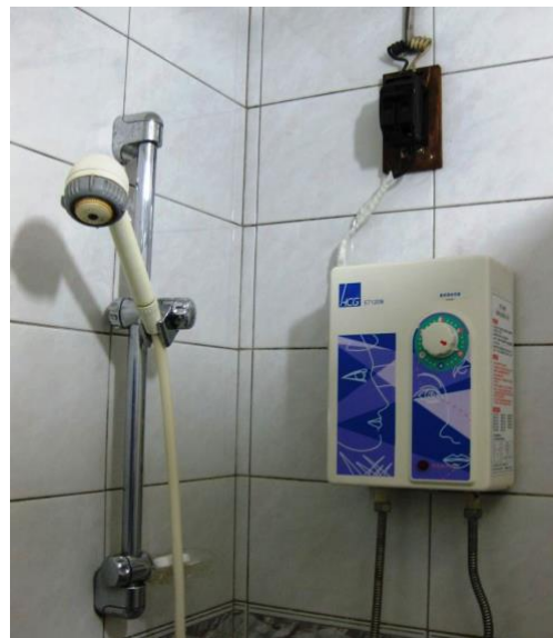
Electric water heater in a shower stall
