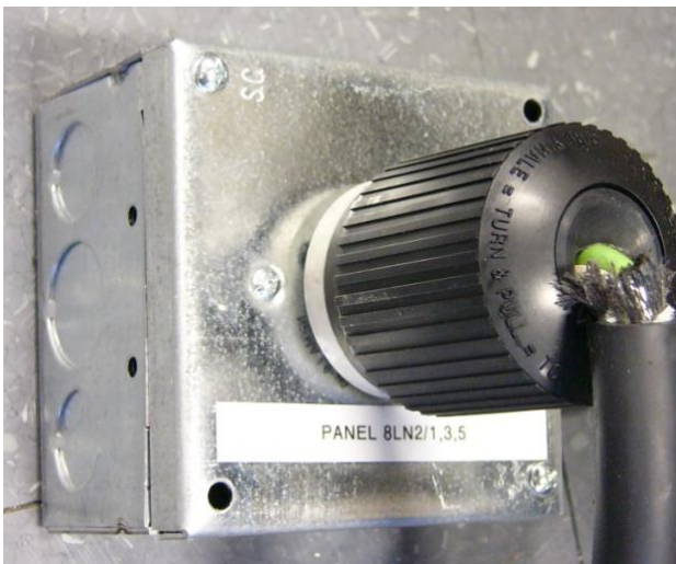
Cord cap needs repair and strain relief
